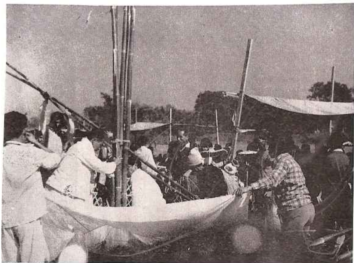
Fixing of the tallest bamboos called PIRSIKPI at the centre of the LANGTUK.
